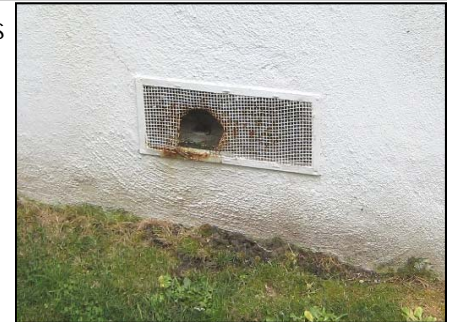
Roof rats can access homes through holes in vents as small as the diameter of a quarter.
