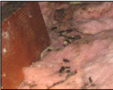
Rat droppings in an attic
